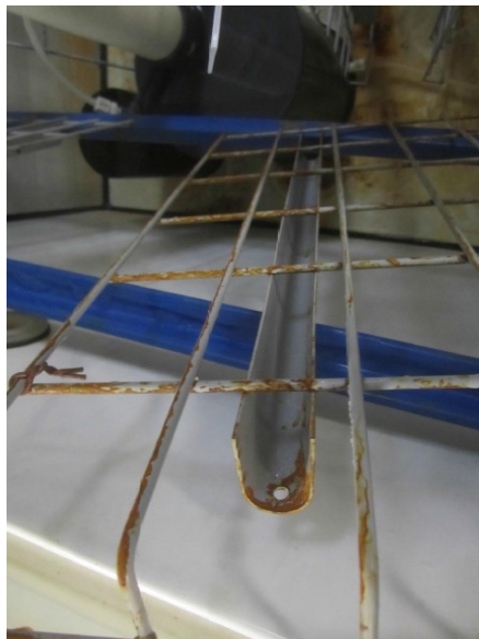
PAINTED DECK (Red Rust Visible)
