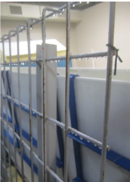
POWDER-COATED DECK (Red Rust Visible)
