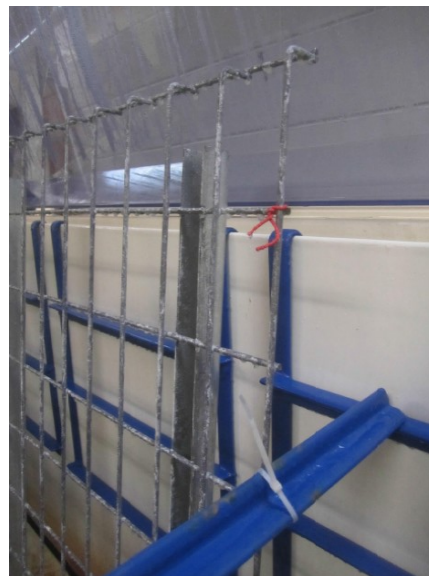
ZINC-COATED DECK (White Rust Visible)
