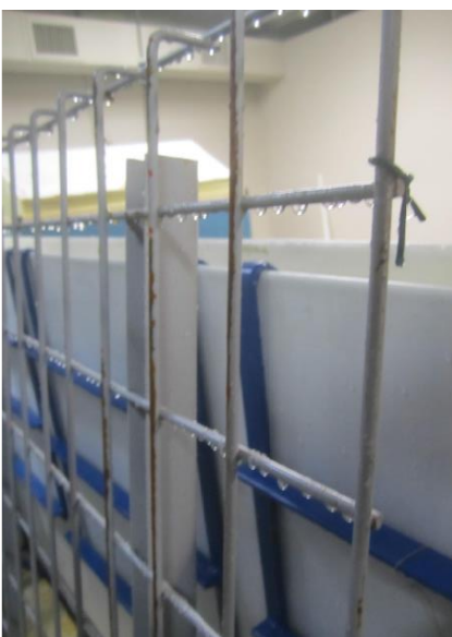
POWDER-COATED DECK (Red Rust Visible)
