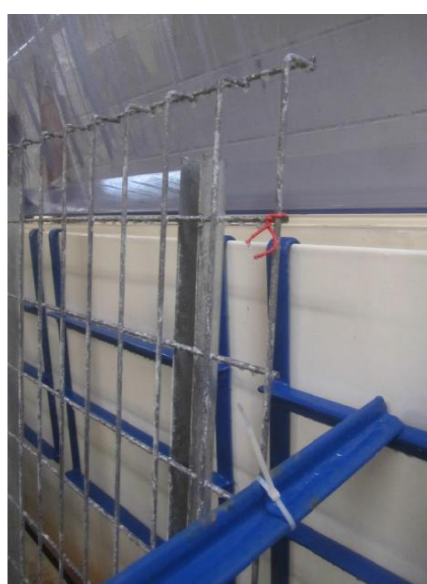
ZINC-COATED DECK (White Rust Visible)
