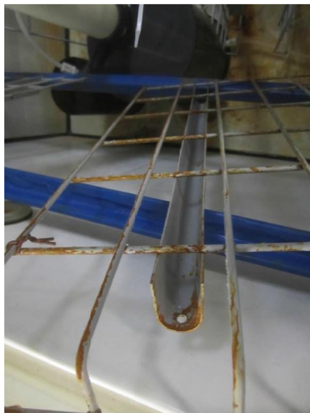
PAINTED DECK (Red Rust Visible)
